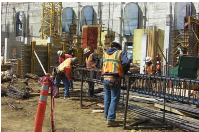
Instead of having ironworkers bend to tie rebar, the work is raised to their comfort zones. Courtesy, Occupational Health Branch, CDPH
